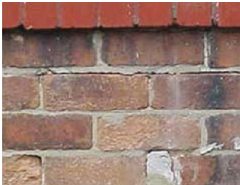
Fig4—Horizontal cracking in mortar joint
