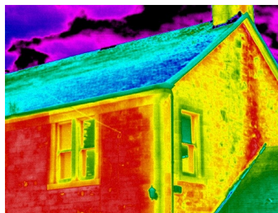
Thermographic image showing heat loss
